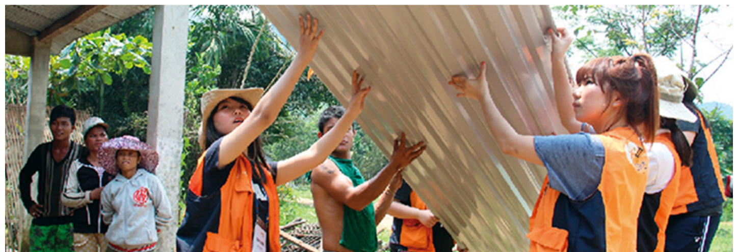
Volunteers from Hanwha help install a corrugated roof on a donated charity house in Quảng Điền District, Thừa Thiên-Huế Province
